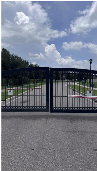
Gate misalignment at closing edge
