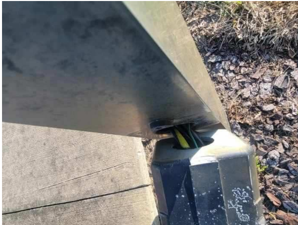
Pull box broken off at button pole
