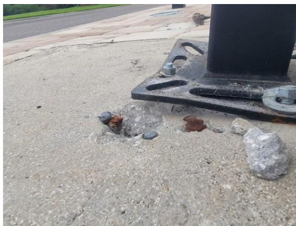
Bent pedestal base before remounting
