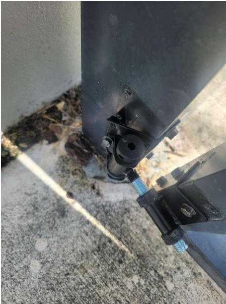
Pedestrian gate lower hinge — replacement needed
