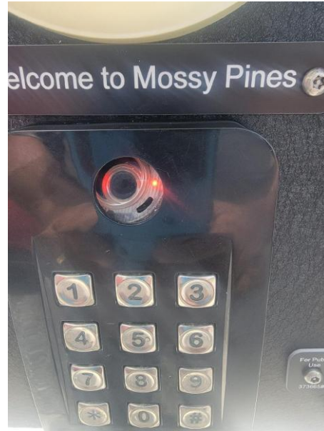
Access keypad — struck; scheduled for replacement
