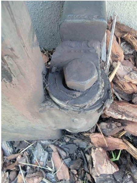
Broken bottom hinge at exit gate
