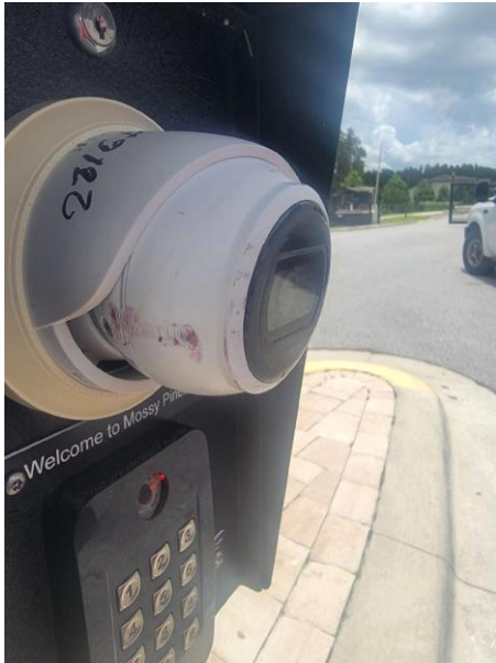
Pedestal camera and telecom reader
