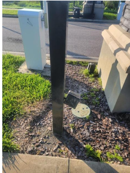
Pull box location — exit pedestrian gate
