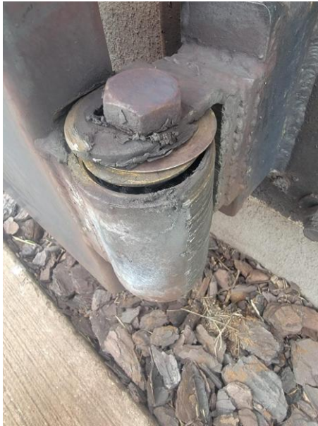
Broken bottom hinge at entry gate
