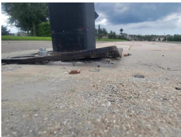
Pedestal base plate bent; anchors pulled from concrete
