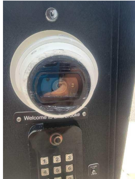
Pedestal camera knocked out of alignment
